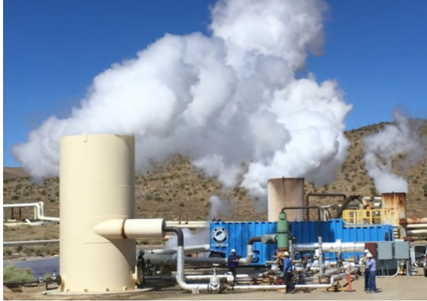
Figure 4: GreenFire Energy's 2019 demonstration project at the Coso Geothermal Power Plant, Coso, CA.
