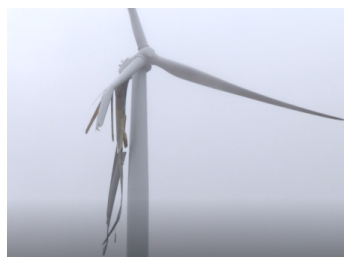
Figure 7.10: Wind turbine damaged by high wind speed.
